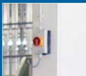
lockable main switch
