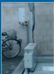
lockable main switch
